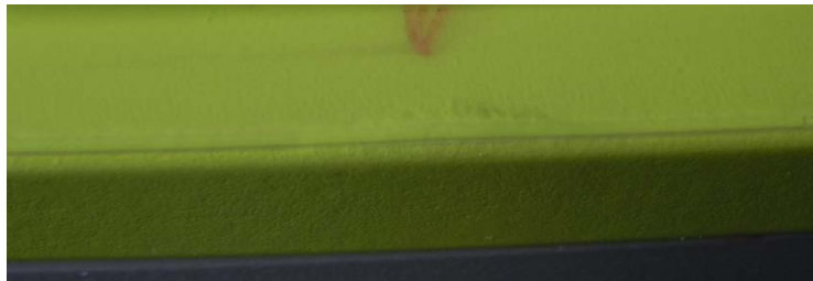
A-I-14 after 6 cycles, swelling of the coating along the edge at one point
